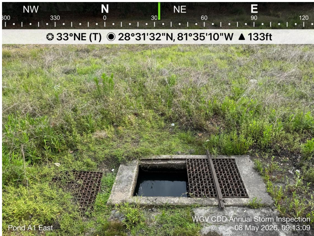
PHOTO #3.2 – Pond A1 East Bubble Up Structure #2 on May 8, 2026
