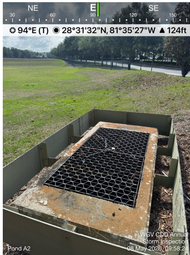
PHOTO #9.1 –Control Structural Weir for A2 on May 8, 2026.
