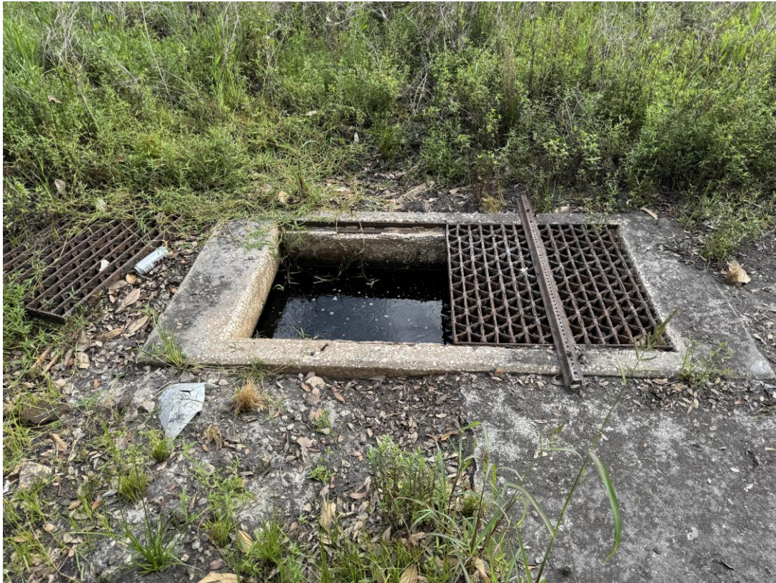
PHOTO #3.1 – Pond A1 East Bubble Up Structure #2 on May 23, 2025
