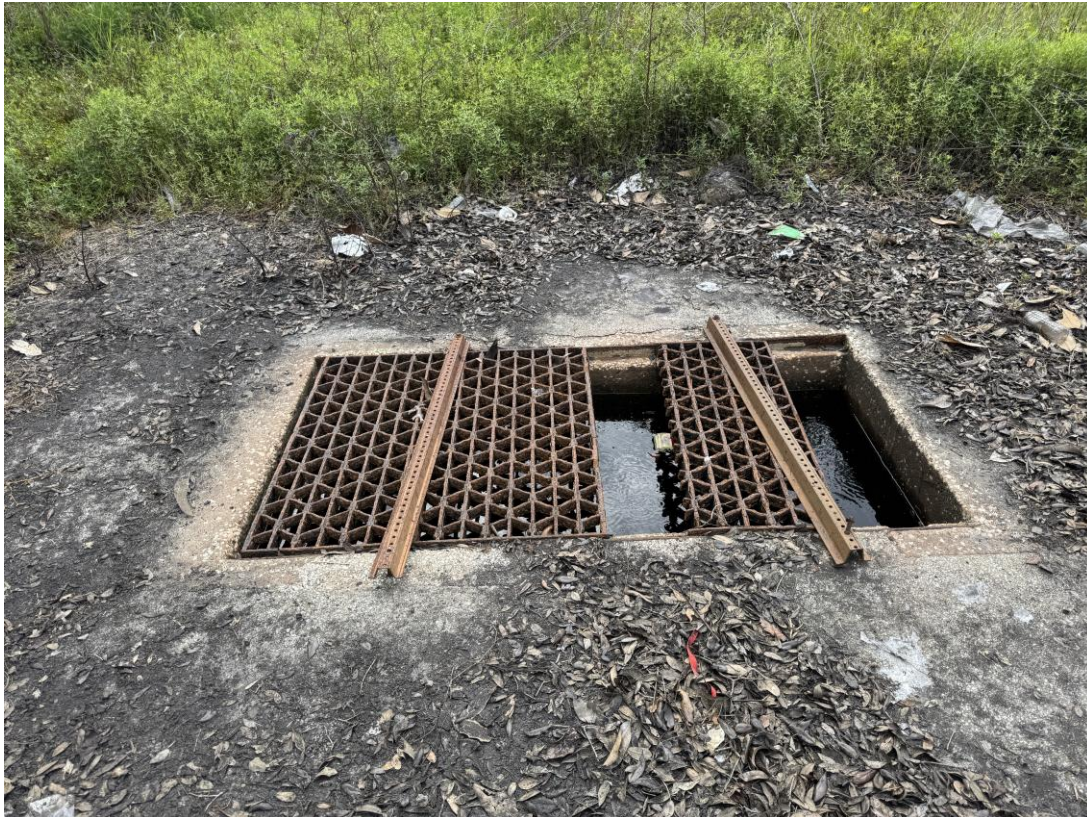
PHOTO #2.1 – Pond A1 East Bubble Up Structure #3 on May 23, 2025
